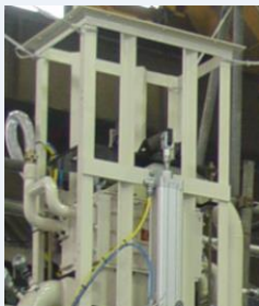
Inter_Cooler Temp Controller
